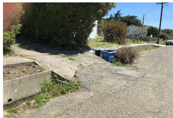
Figure 9: North side Mill Street - challenge at driveways
