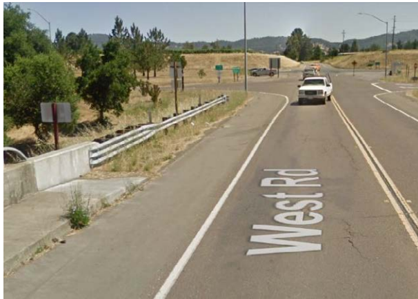
Figure 201: End of Sidewalk on West Road Bridge, looking north (Source: Google Street View)
