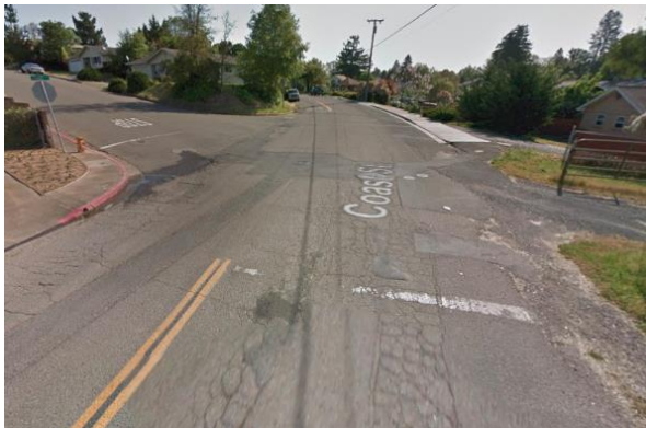
Figure 121: The intersection of Coast Street and Mill Street is lacking ADA accessible curb ramps at three corners (Source: Google Street View)
