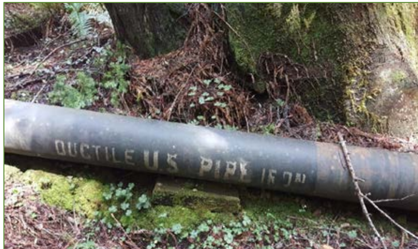
Above-Ground Ductile Iron Pipe
