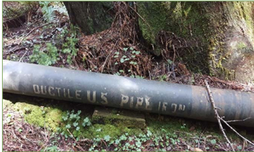
Above-Ground Ductile Iron Pipe
